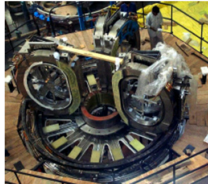
FIG. 4. TF modules on support structure
